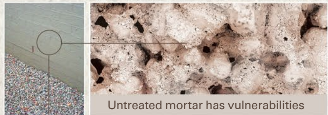
Untreated mortar has vulnerabilities
