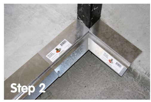
Step 2 The premade Corner cap is positioned over straight lengths of capping to form internal or external corner.
