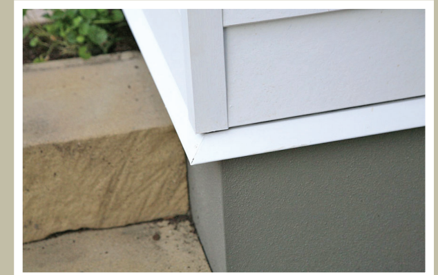
The use of pre made corners saves on site manufacturing time of up to 30mins per corner for carpenters.
